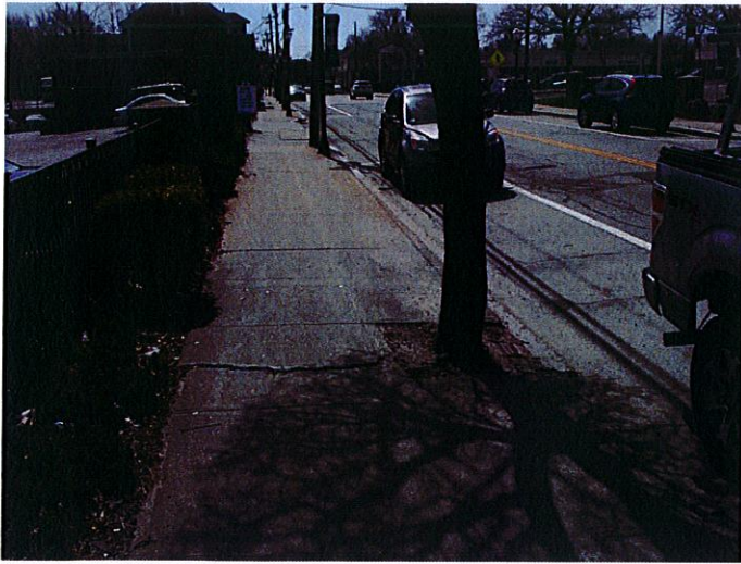
Tree well and cracked sidewalk near 500 Main Street prior to improvement
